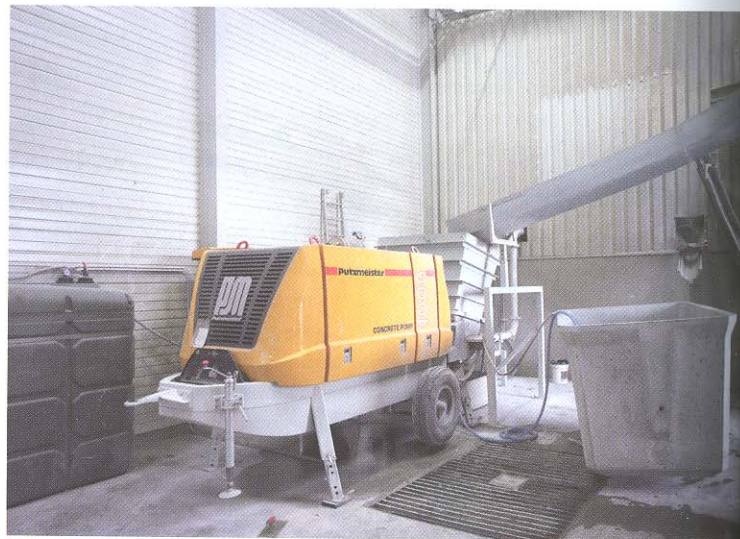
The stationary Putzmeister BSA 1005 concrete pump is responsible for conveying concrete by pipeline (DN 100) to both places of production
