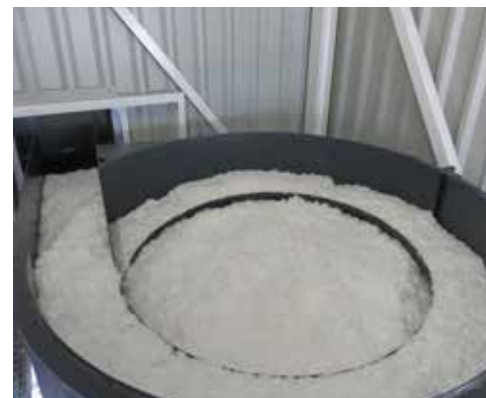
Dosing unit model MD400 installed in Switzerland 2015.
